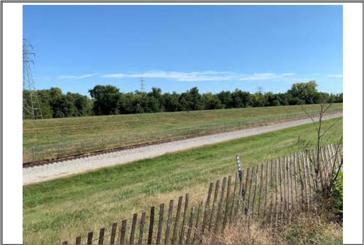
Photograph Number 9: The Wood River Creek Levee comprises the east side of the property. Facing southeast
