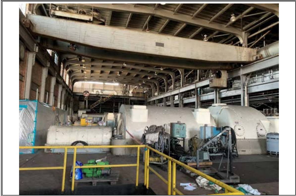
Photograph Number 13: Power Plant interior (turbine room). Facing East.
