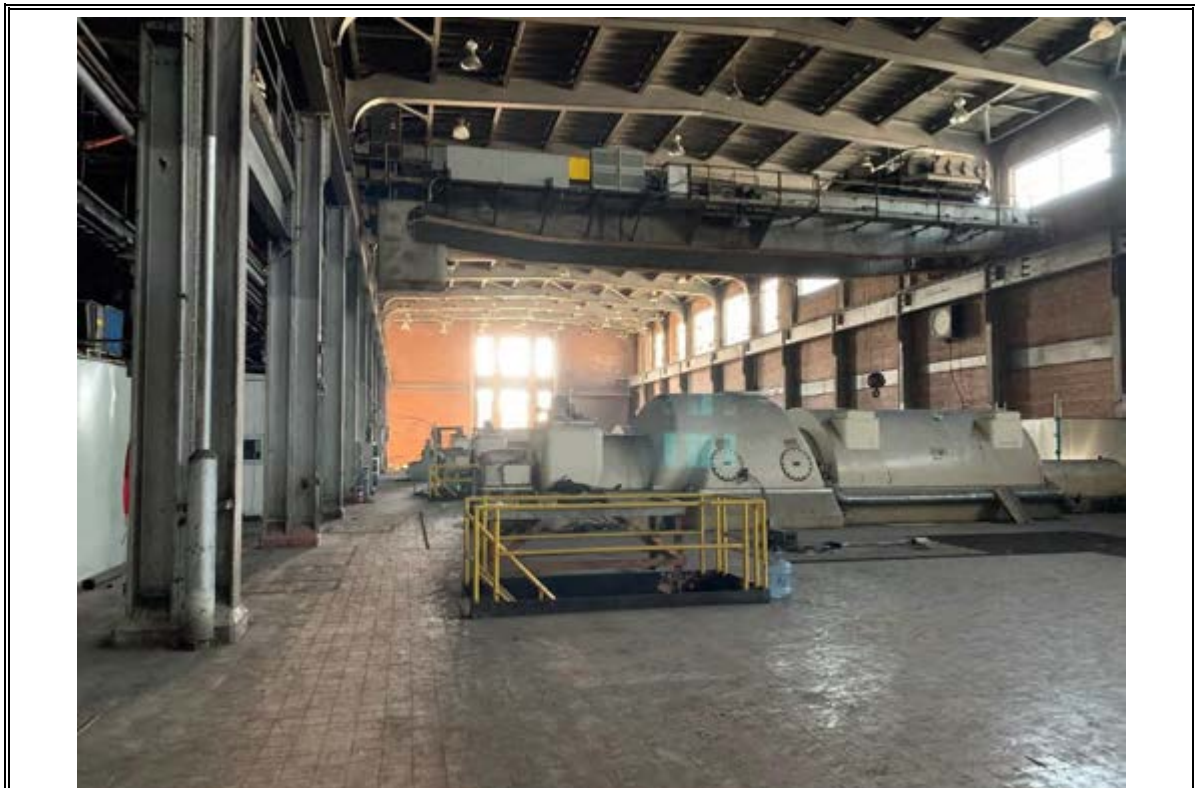
Photograph Number 14: Power Plant interior (turbine room). Facing West.
