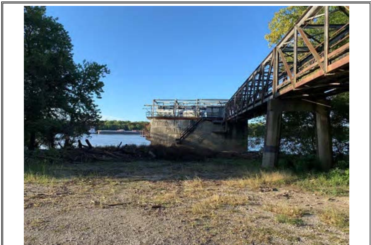
Photograph Number 26: View of the 1 st of two structures expanding south over both levees and IL 143 that concludes at the Mississippi River.
