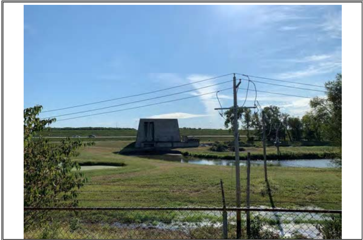
Photograph Number 19: Main pump station building, IL Route 143, and the Mississippi levee. Facing South.
