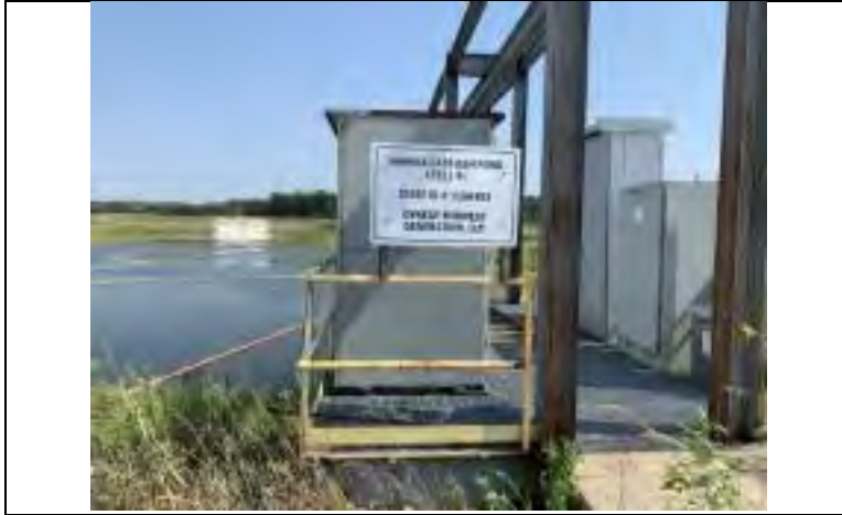
Stormwater Pond (identified as Cell 4)
